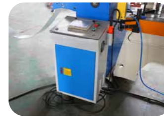
PLC 控制柜 PLC Control Cabinet
